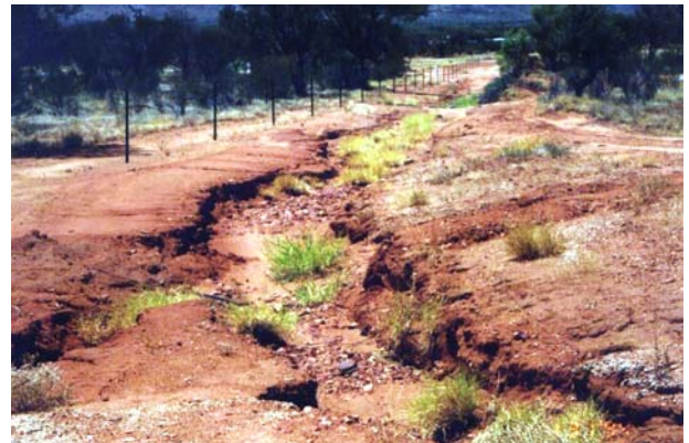
Fence line erosion
