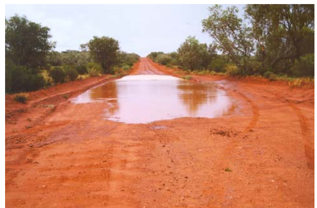
Windrows present – water unable to flow its natural path
