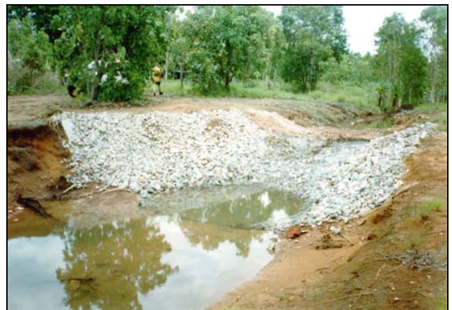
Plate 2 Major drop structure constructed from loose rock held in place by wire netting. Note stilling basin in the centre of the picture
