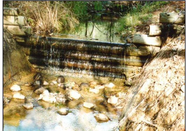
Plate 1 Major drop structure made of logs. Note the concrete and rock apron, and the concrete keying the logs into the side
